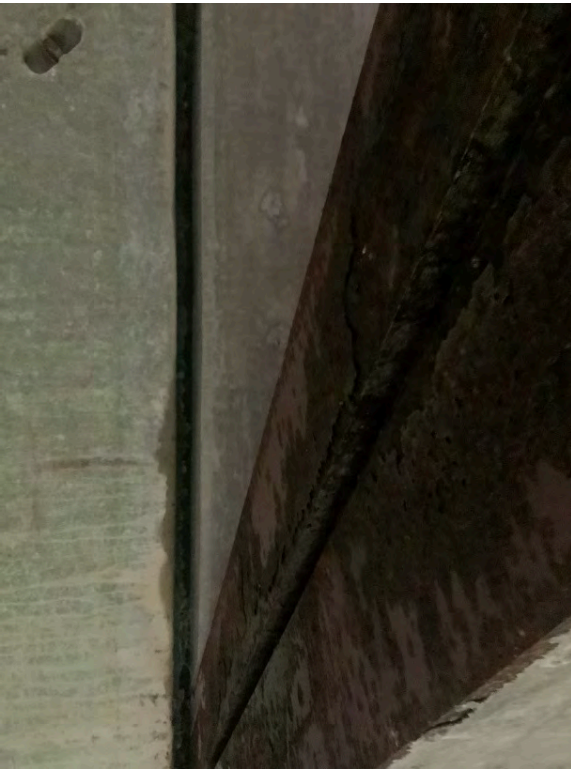
Rust scale bottom of girder
